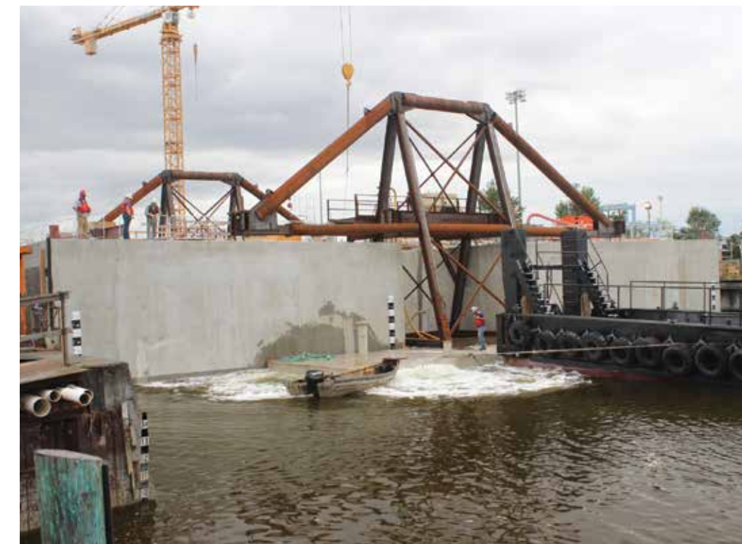
Two pontoons are floated out of the casting basin at Tacoma's Concrete Technology Corp. on the Blair Waterway. Photo courtesy of the Washington State Department of Transportation.
